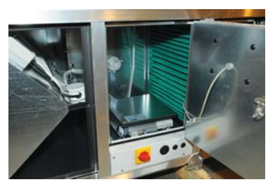
Internal view of "EASY" technical compartment
