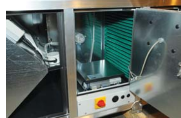
Internal view of "EASY" technical compartment
